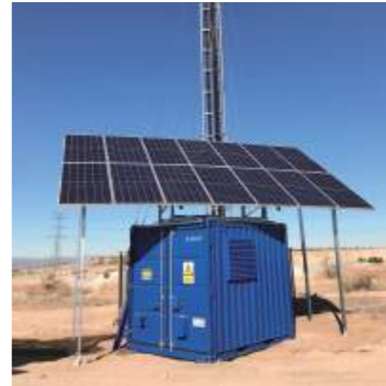
Remote Town in Xinjiang 150kw/200kwh
