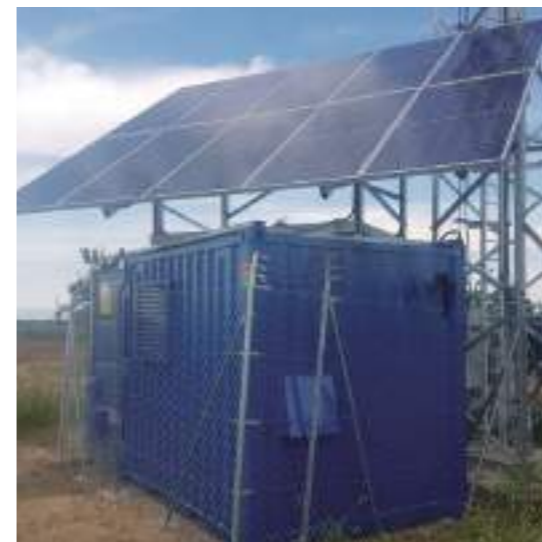
United Arab Emirates 100kw/200kwh
