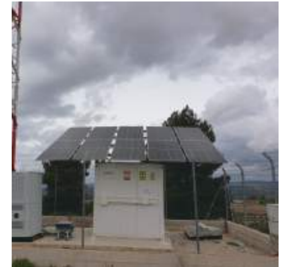
Western Sichuan 60kw/200kwh
