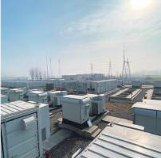
Langfang, Hebei 150kw/306kwh
